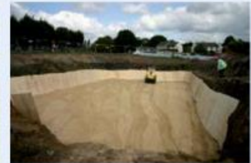
Stage 2: Protect the integrity of the root barrier membrane with a layer of sand and provide shutter ply supports for the edge of the cell.
