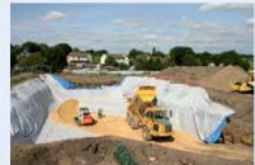
Stage 4: Protect the root barrier membrane from tyre damage with a layer of sand.
